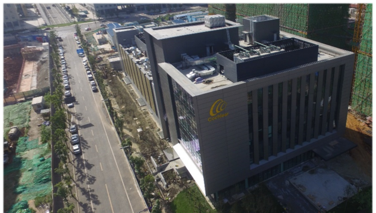
Construction of Cochlear's China manufacturing facility to be completed by the end of 2020
